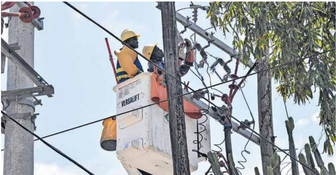
Kenya Power personnel from the Live Line Team near Pandya Memorial Hospital in Mombasa on November 10, 2022. Procurement of metres and transformers has been riddled with accusations of corruption.
